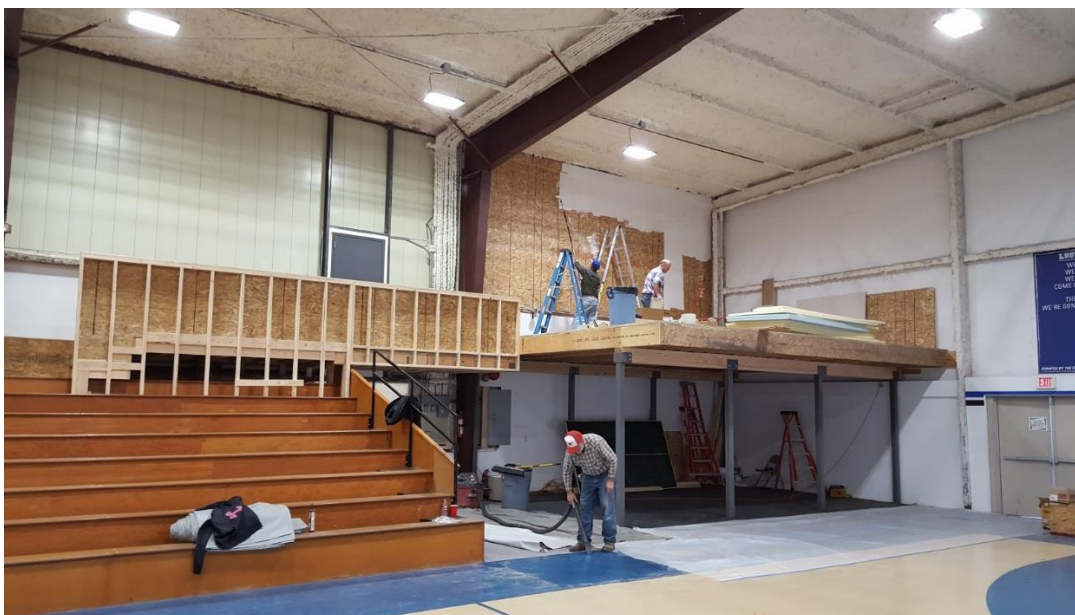
Work being done to build the mezzanine which will give convenient access to the assembly room. Photo by Becca Reddig
